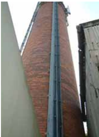
Cable management running up chimney stack
