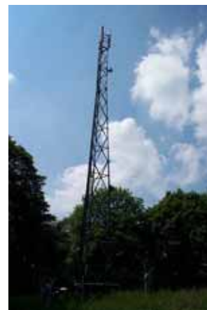
Site share lattice tower
