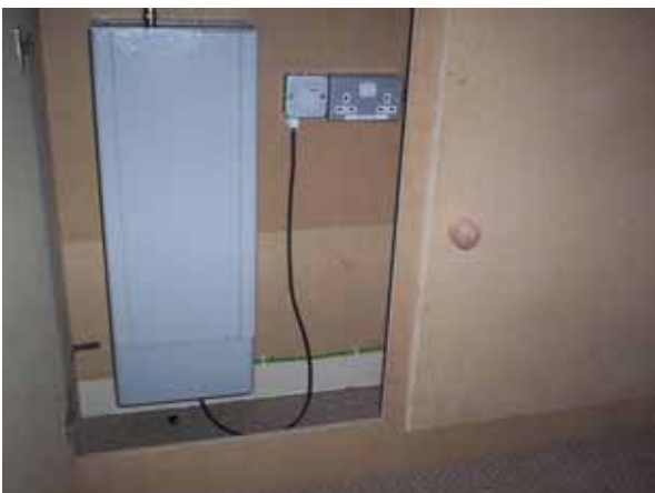
Radio frequency equipment installed in cabinet
