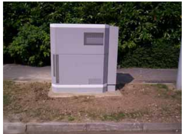
Upgrade of UMTS equipment - after
