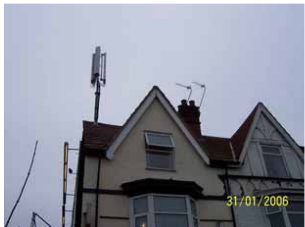
Antenna mount located through roof into building
