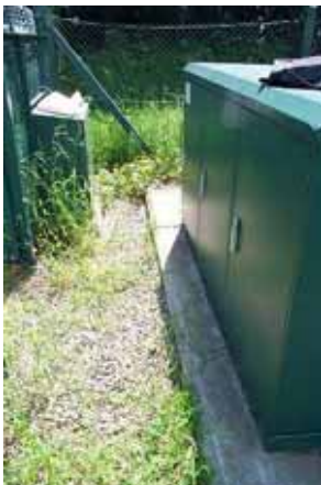
Site share equipment cabinet
