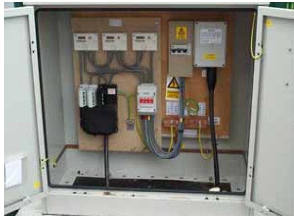
Site share meter cabinet
