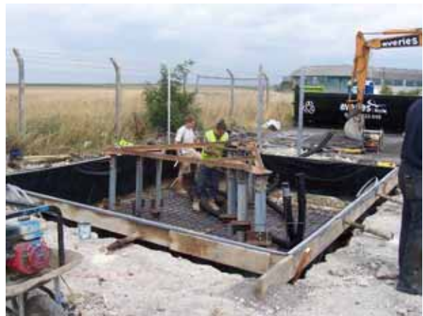
Greenfield macro tower base
