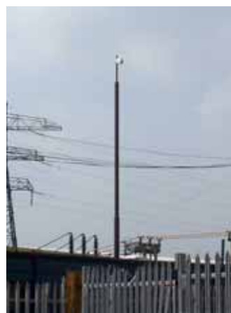
Microwave dish mount structure
