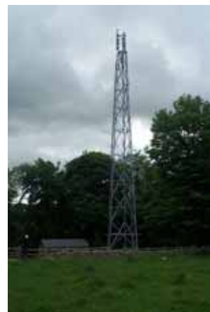
Site share lattice tower
