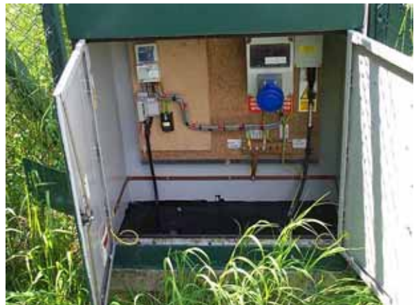
Site share meter cabinet
