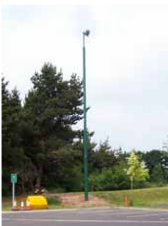
Microwave dish mount structure
