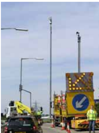
Microwave dish mount structure
